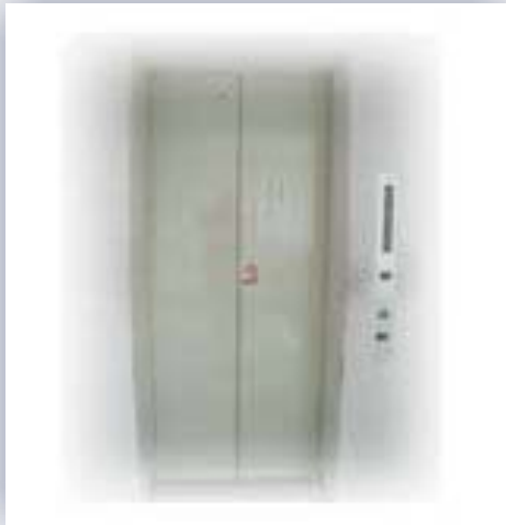
2 high speed passenger lift and 1 stretcher lift
